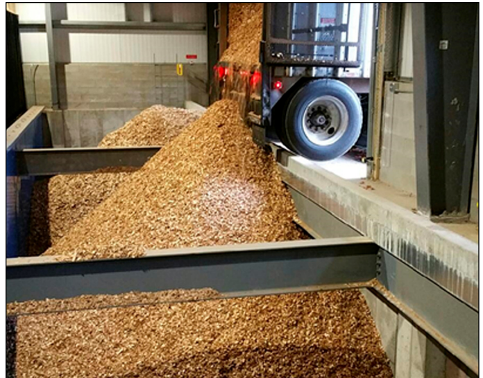
The biomass fuel storage bunker holds up to 120 tons of wood chips that can provide heat to the campus for up to three days.
